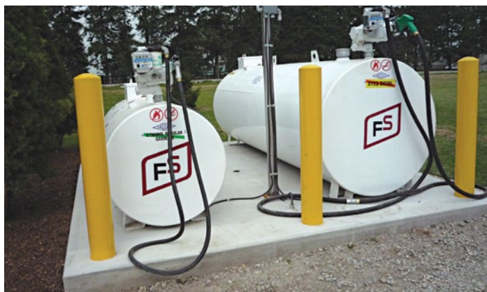
Figure 2.1. On-farm fuel storage with vehicle protection (bollards).
