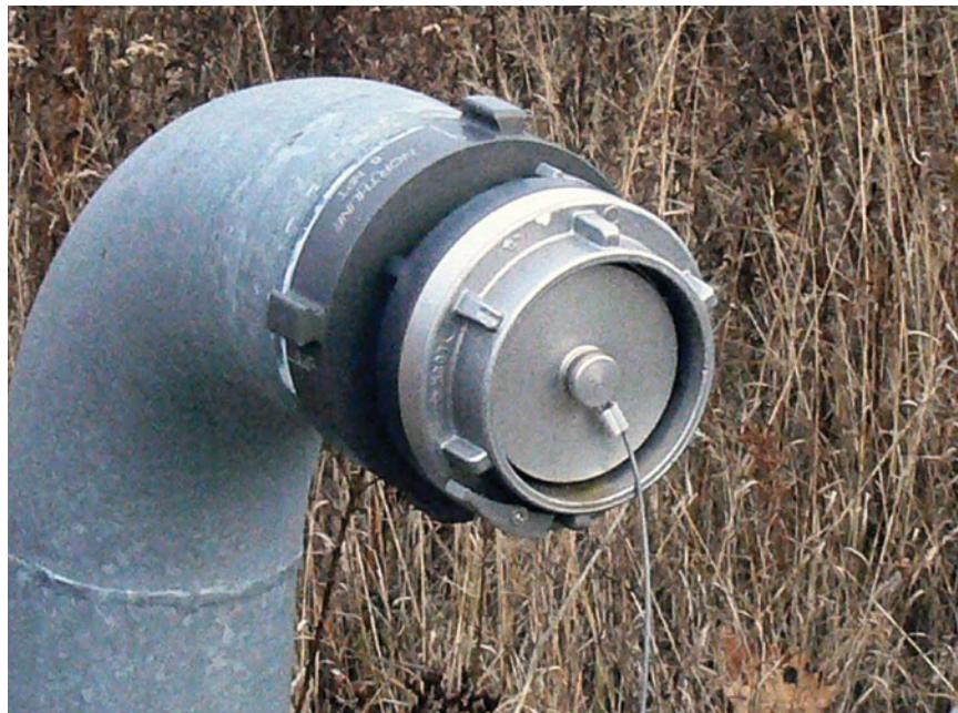
Figure 4.6. Dry hydrant standpipe connection.
